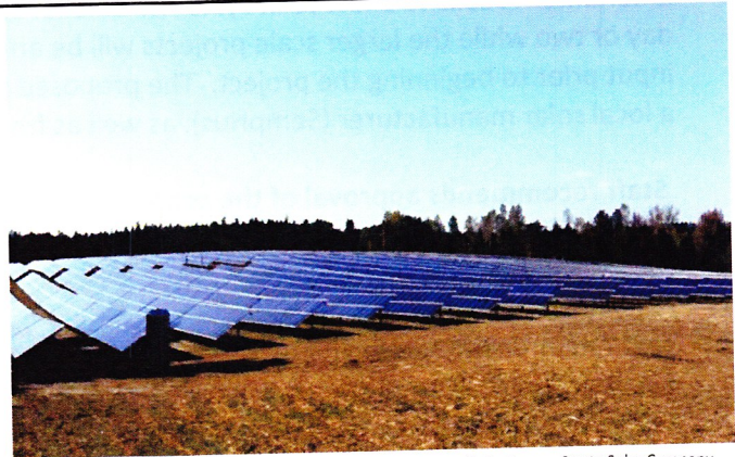
Warren County Solar Farm – Strata Solar Company
